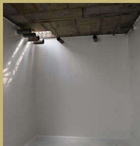
06 WATER TANK FOOD GRADE TREATMENT
