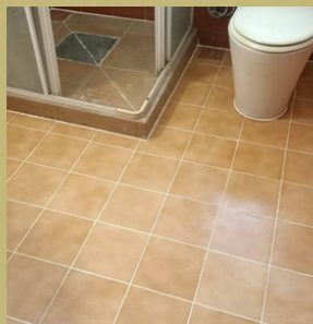
04 LEAKY TILED TOILETS WP
